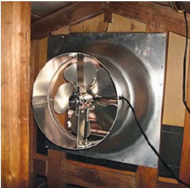
gable mounted fan (view from inside attic)
